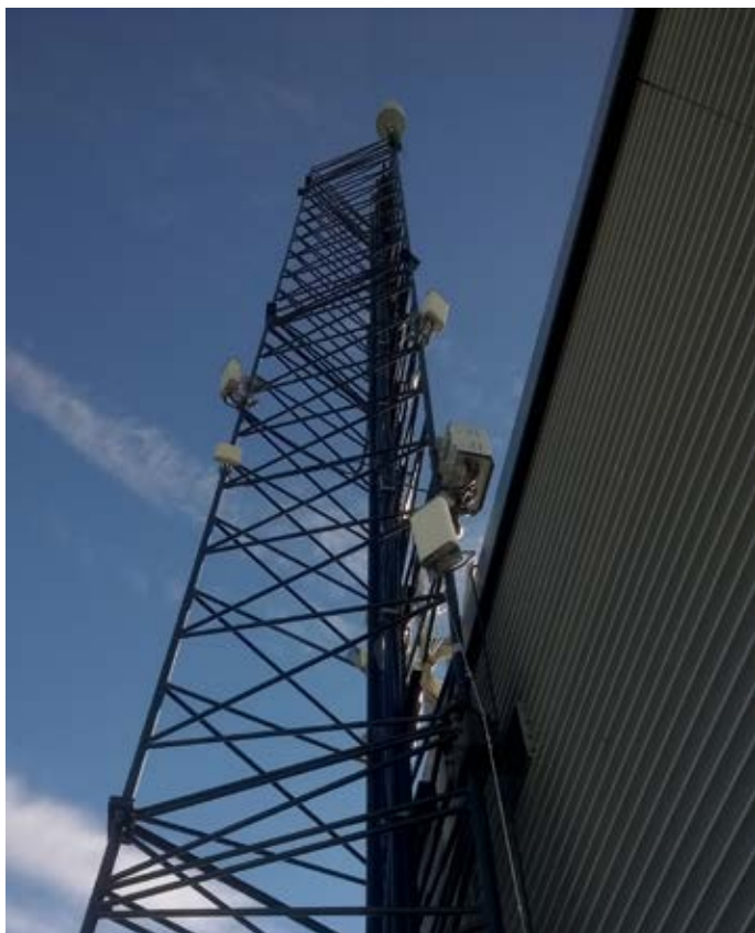
Kuva 4. Oulun yliopiston 5G-testiverkon makrosolun masto. Figure 4. Macro cell tower in 5G test network at University of Oulu, Finland.
